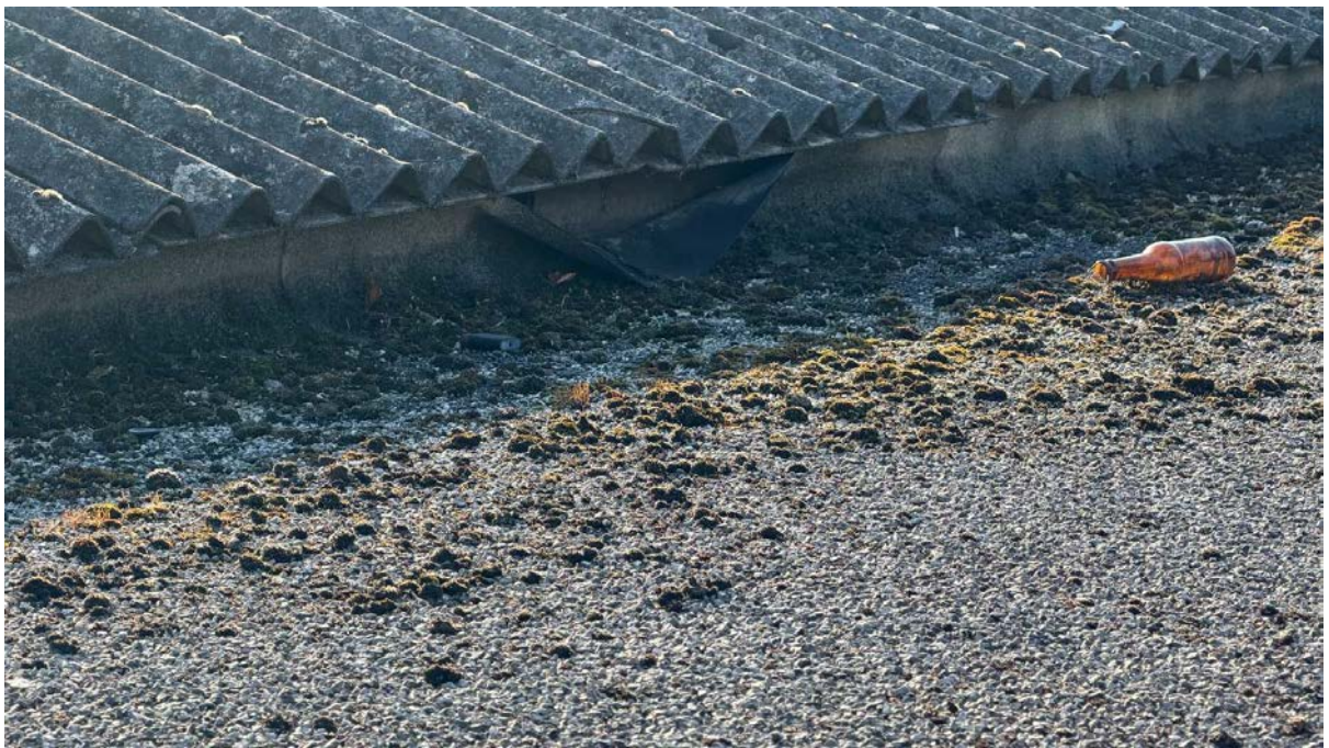
Area of slipped roof felt.
