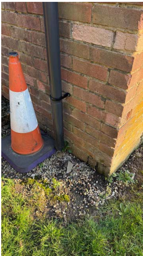
Downpipe exit out onto earth around main walls.
